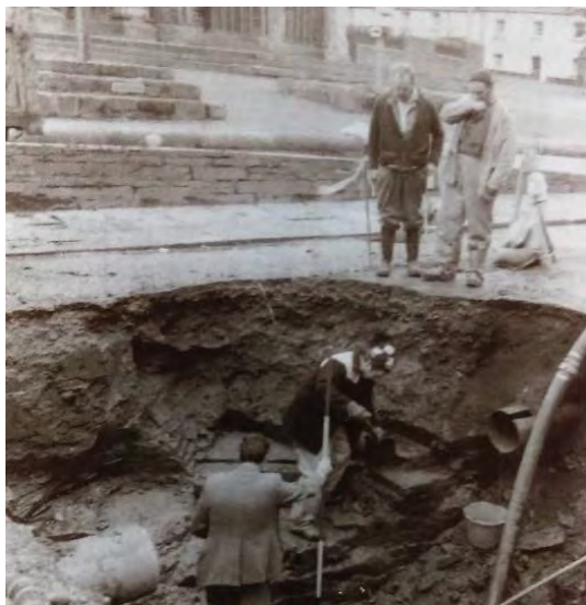
Fig 7: Sump hole being dug on Broad Street outside the cathedral in 1986. The ranging pole at the vertical base of the rock cut. Image National Monuments record of Scotland (1986)
